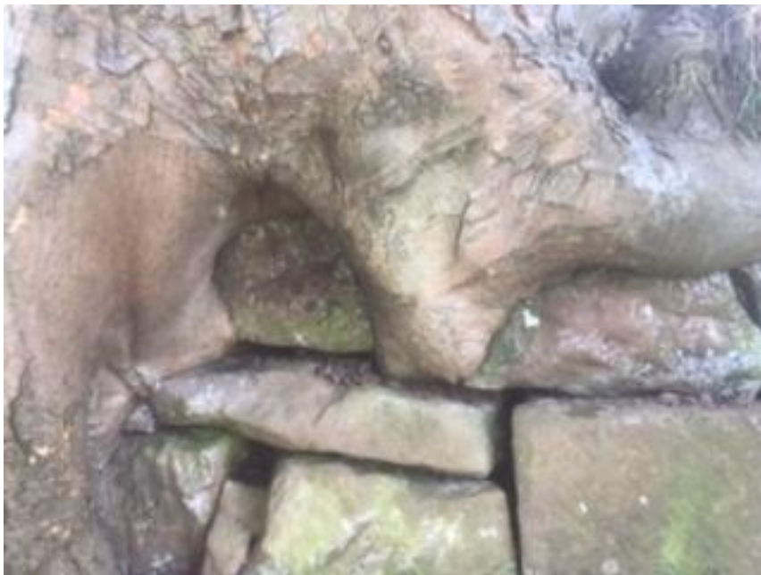
Sycamore in dam wall
