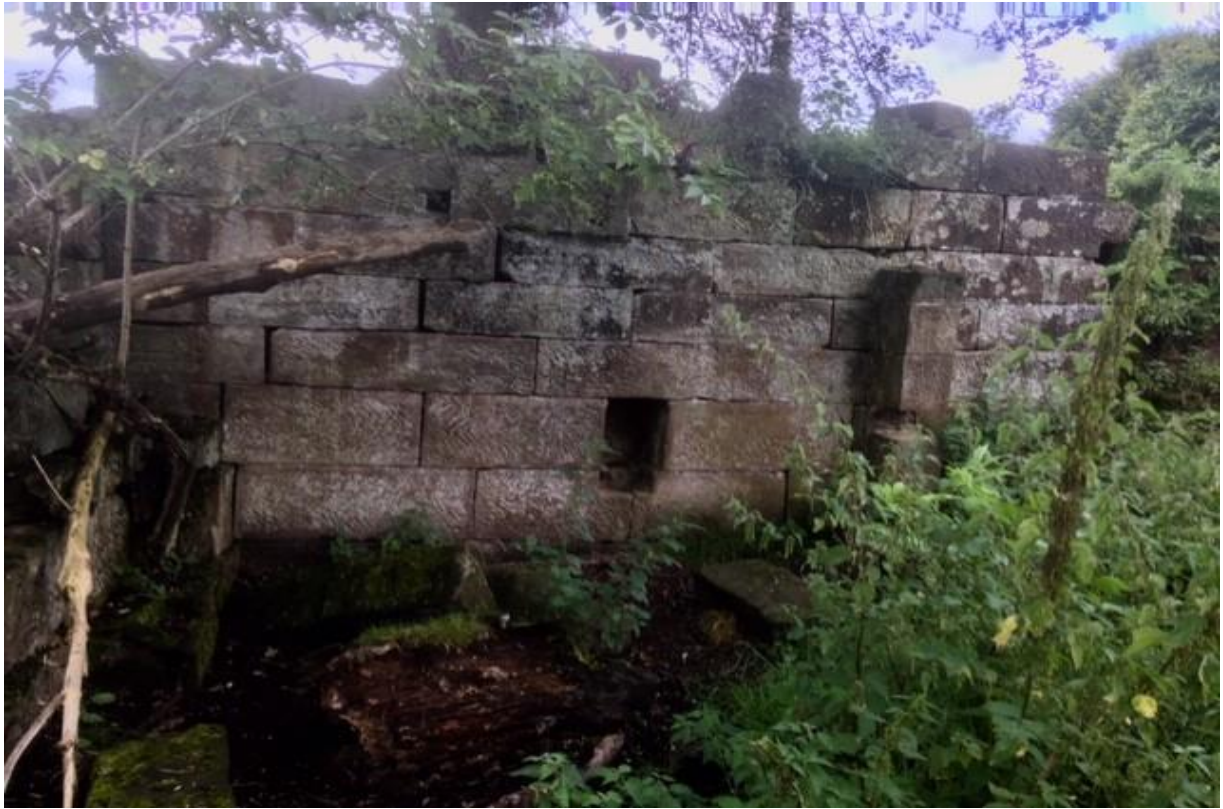
Mill backwall showing two small floor joint holes
