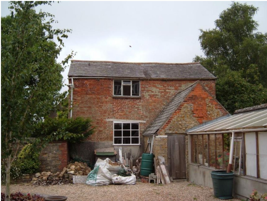
The stables and bothy. There were three stalls and probably room for a cart. The single storey extension was the bothy for the stable lad where there was a bunk and small stove. The water would be drawn from a well the other side of the mill.
